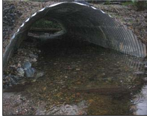
Photograph 17. Example of a fish-friendly culvert (photograph courtesy of Mid Puget Sound Fisheries Enhancement Group).
