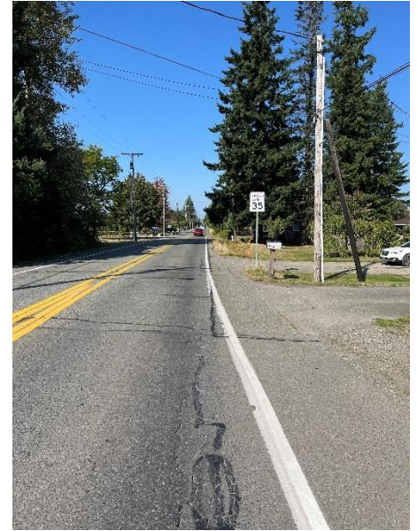
Figure 14-Northbound Porter St lack of active transportation facilities
