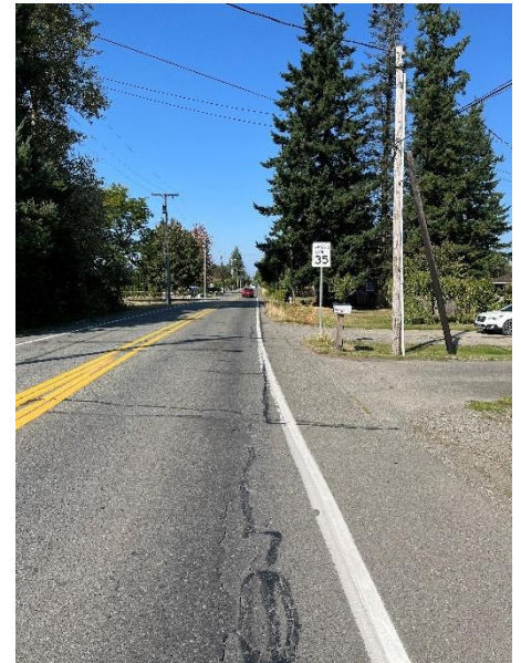
Figure 14-Northbound Porter St lack of active transportation facilities
