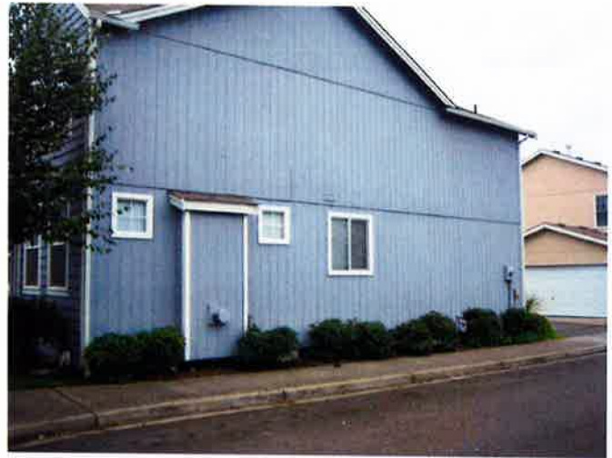
Figure 4-14. T-111 siding is prohibited.
