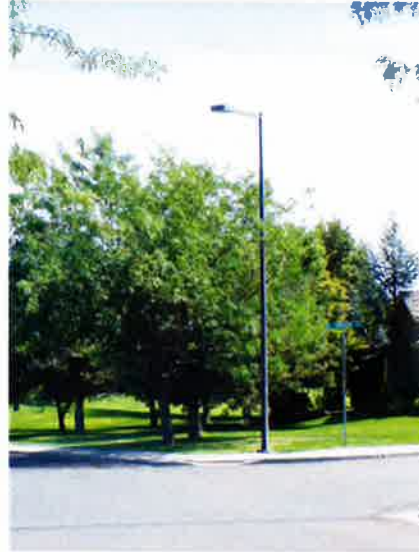
Street light at Canyon Lakes
